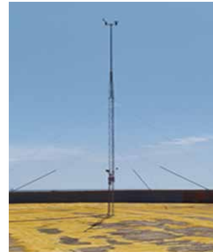
1. New East Breakwater Weather Station
